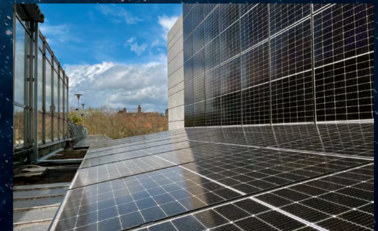
Cinecitta's roof areas are covered with 800 photovoltaic modules
